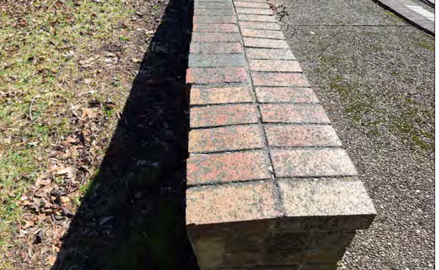
LOCATION G - FULL BRICK REPLACEMENT ALONG TOP OF WALL DUE TO MISMATCHED BRICK SIZES AND COLORS.
