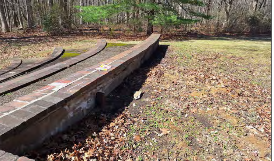
TYPICAL CONDITION - LOCATION I - FREESTANDING WALL PACKING REPAIR. REPLACE UNEVEN, FAILING PAVING ALONG REAR OF FREESTANDING WALL.
