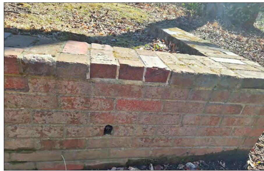
TYPICAL CONDITION - LOCATION A: INDIVIDUAL BRICK REPLACEMENTS ASSOCIATED WITH CHIPPED/DAMAGED/MISMATCHED BRICKS AND ELECTRICAL WALL PLATE REMOVAL, ON HORIZONTAL AND VERTICAL FACES.
