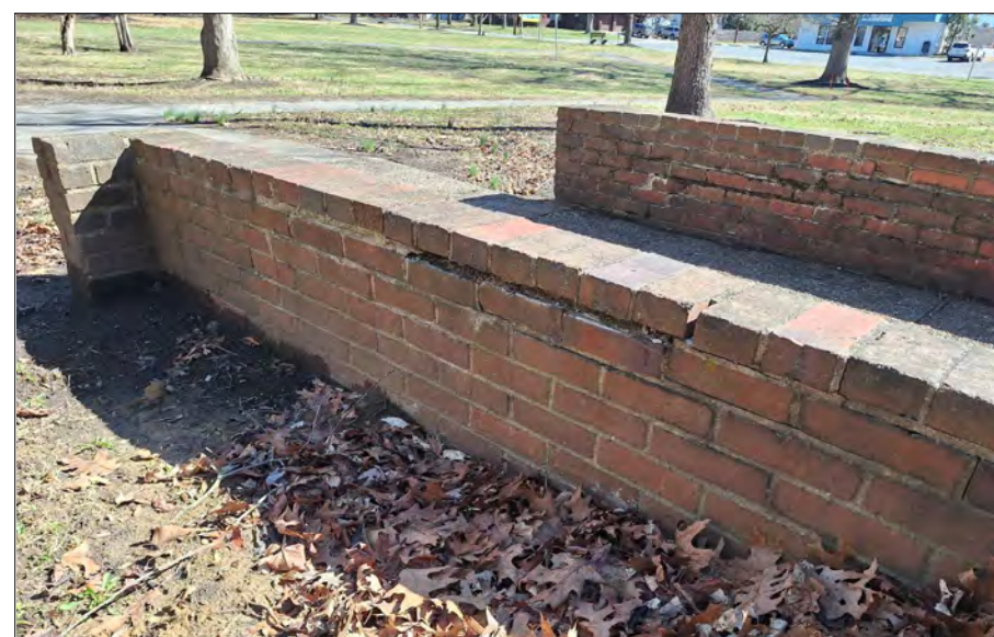
TYPICAL CONDITION - LOCATION F: BRICK REPLACEMENTS ASSOCIATED WITH DEEP MORTAR REPAIR AND REPLACEMENT ALONG FREESTANDING BRICK WALL SECTION.
