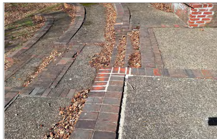
TYPICAL CONDITION - LOCATION E: BRICK REPLACEMENTS ASSOCIATED WITH PREVIOUS MISMATCHED BRICK REPLACEMENTS ALONG WALL SECTIONS.
