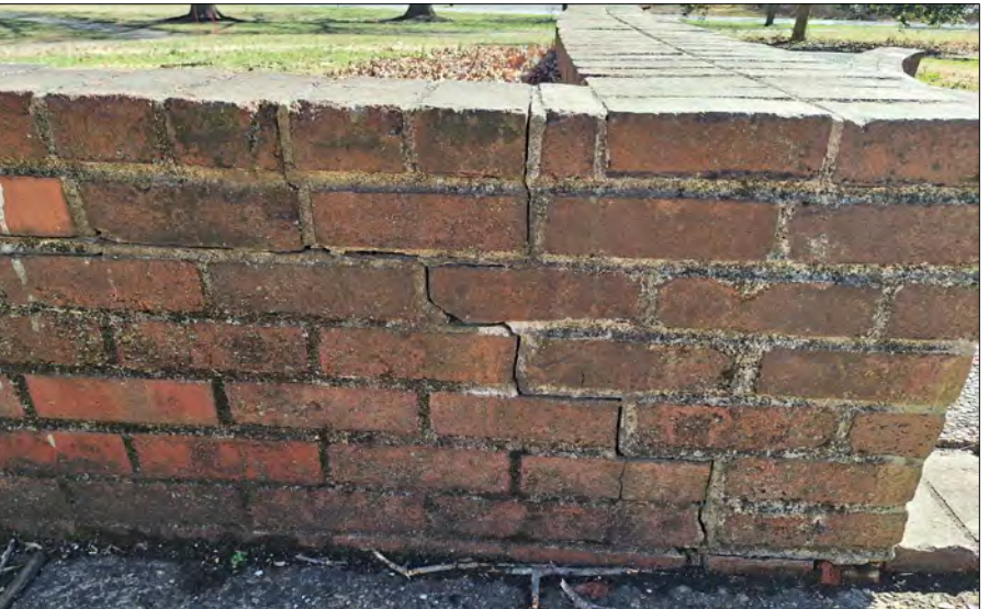
TYPICAL CONDITION - LOCATION H: MORTAR REPAIR AND SELECTIVE BRICK REPLACEMENTS ASSOCIATED WITH STAGGERED CRACK ALONG FREESTANDING BRICK WALL SECTION.
