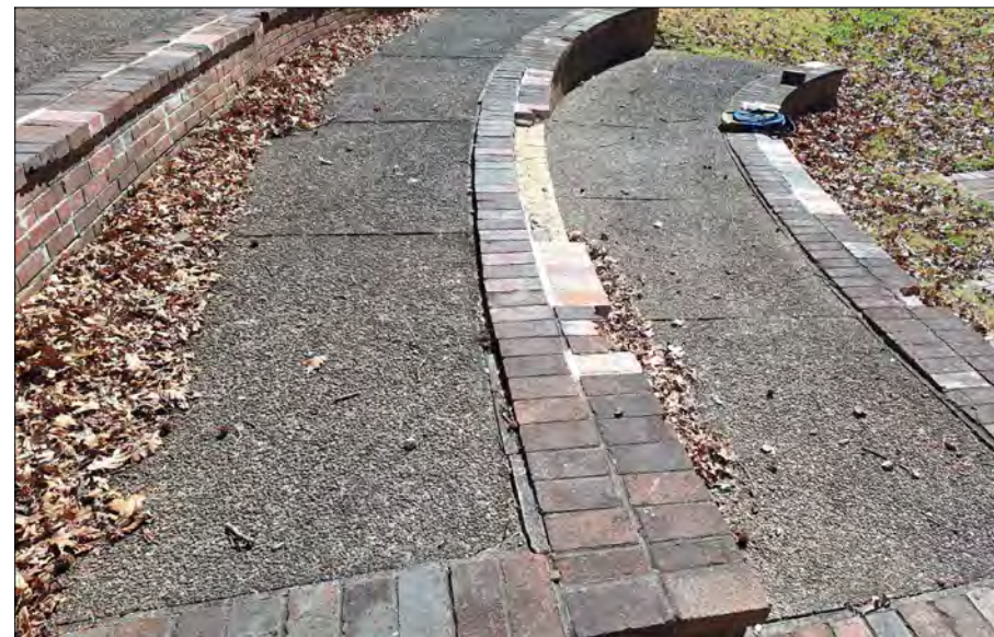
TYPICAL CONDITION - LOCATION D: BRICK REPLACEMENTS ASSOCIATED WITH CHIPPED/DAMAGED/LOOSE BRICKS ON HORIZONTAL FACES.
