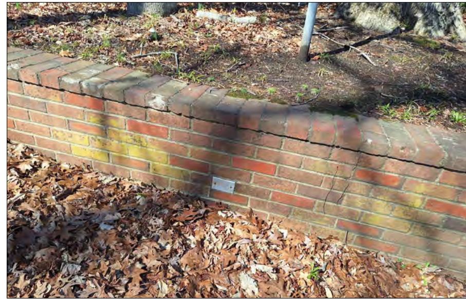
TYPICAL CONDITION - LOCATION B: INDIVIDUAL BRICK REPLACEMENTS ASSOCIATED WITH CHIPPED/DAMAGED/MISMATCHED BRICKS AND ELECTRICAL WALL PLATE REMOVAL (SHOWN), ON HORIZONTAL AND VERTICAL FACES.
